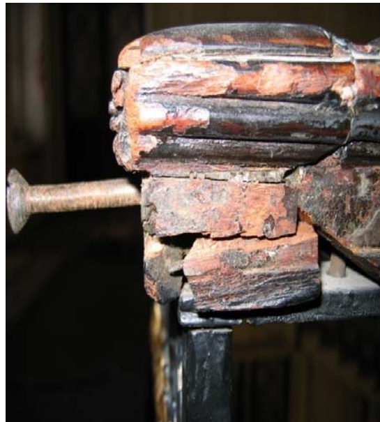
Damage to the handrail corner including an old repair.
